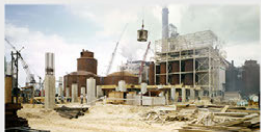
Jesup plant expansion makes it the largest kraft pulp production facility in the world
